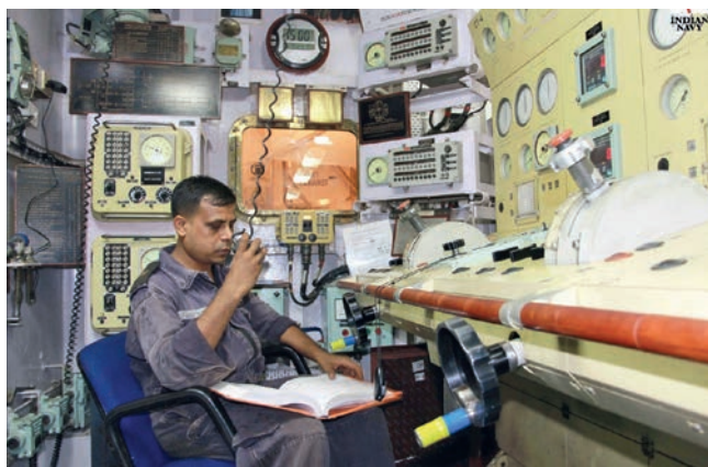
Keeping an Eye on the Machinery
